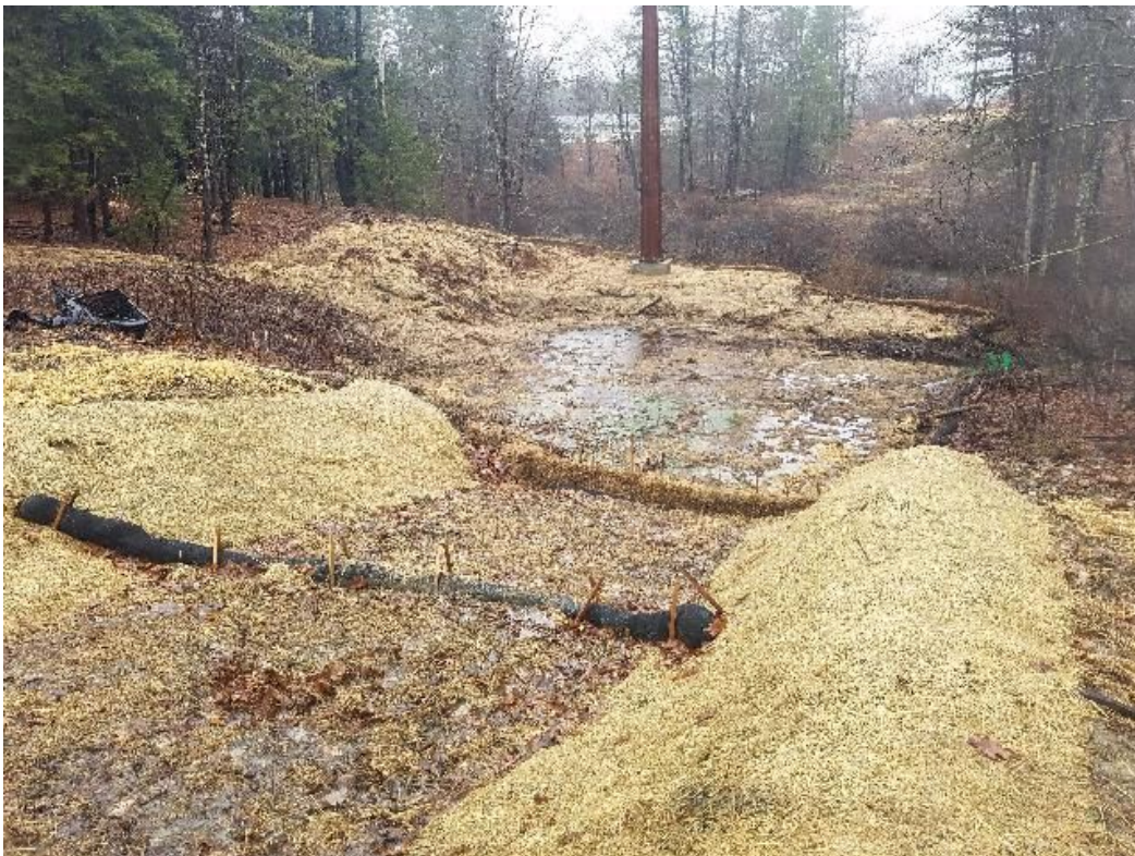
Fig 14: Access road to Str. 28. Viewing north. (04-03-20). Repairs made on 04/01/20 are effective.
