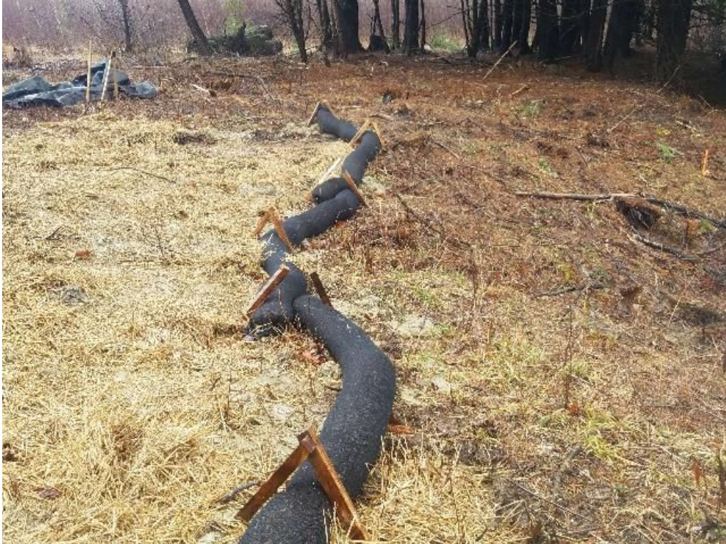
Fig 7: Sediment undercut filter sock at Str. 51. Add additional filter sock. Viewing west. (04-03-20).
