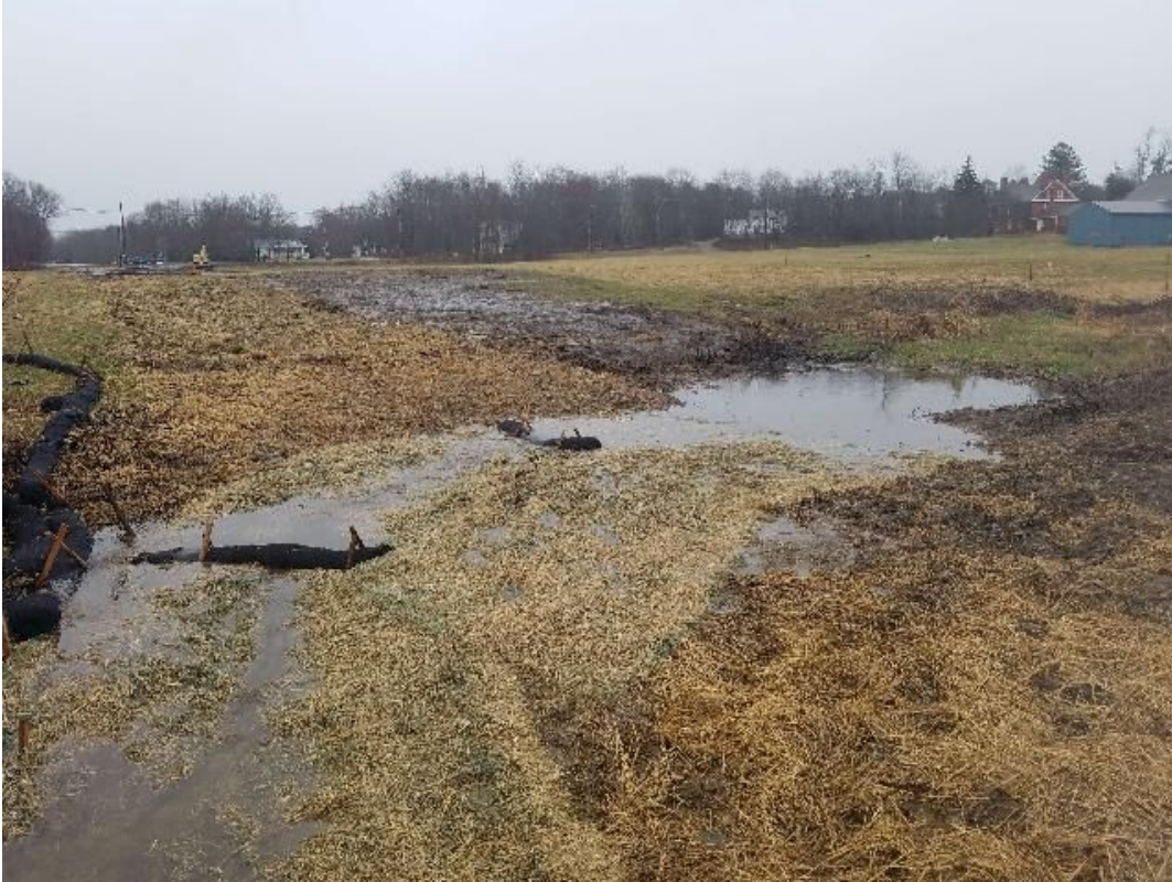
Fig 3: Wetland NW18 at Frink farm. Viewing east. (04-03-20). Repairs made on 04/01/20 are effective.
