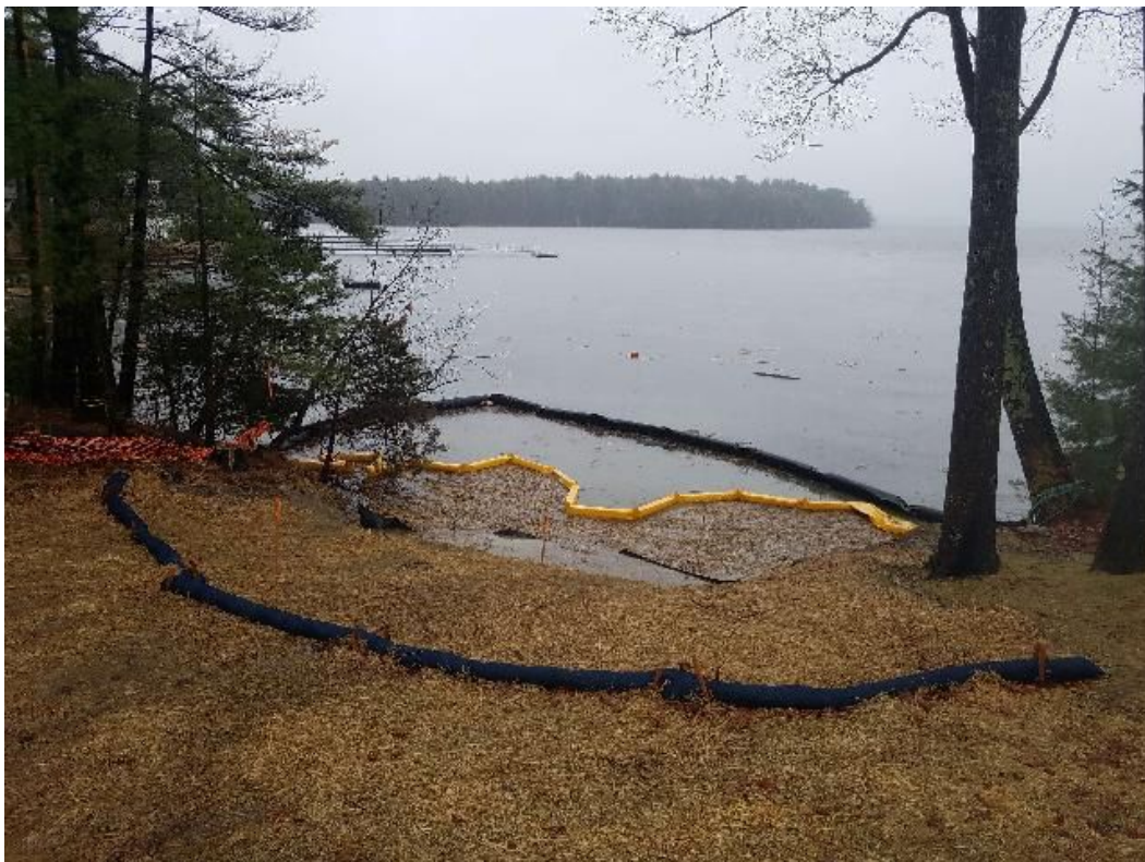
Fig 2: Turbidity curtain in intertidal zone at Gundalow landing/east side of the Bay. Viewing south. (04-03-20).
